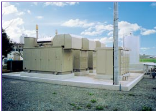
On-site business (In-house electric power)
